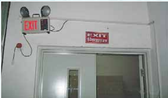
Emergency Light/ Exit Opening Outwards
