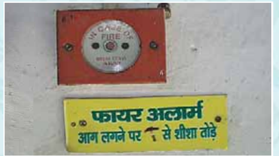
Emergency Fire Alarm Point
